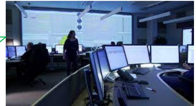
Windfarm and Landfall - Control station
